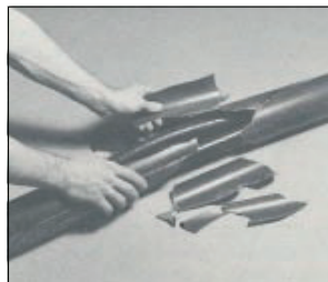
Remove damaged or faulty ducting
